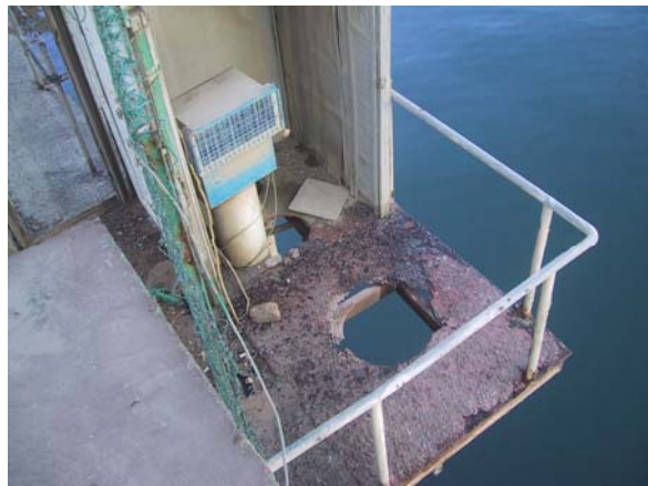
Figure 15, Old Tide Gauge with solar panel (no longer operational), Casablanca.
