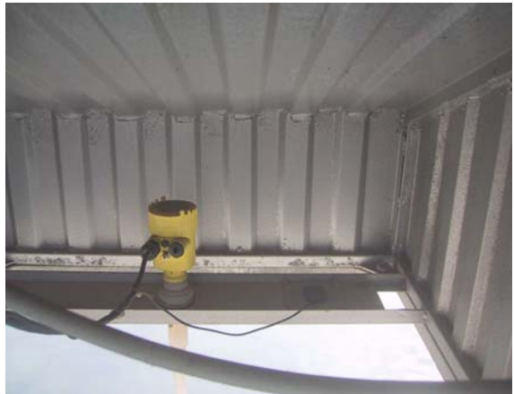
Figure 21, VegaPuls Radar Sensor (yellow) and GPS Patch Antenna alongside at the open base of the galvanised steel cabinet. The microwave/radar antenna wave-guide extends (approx 35cm) below the VegaPuls sensor.
