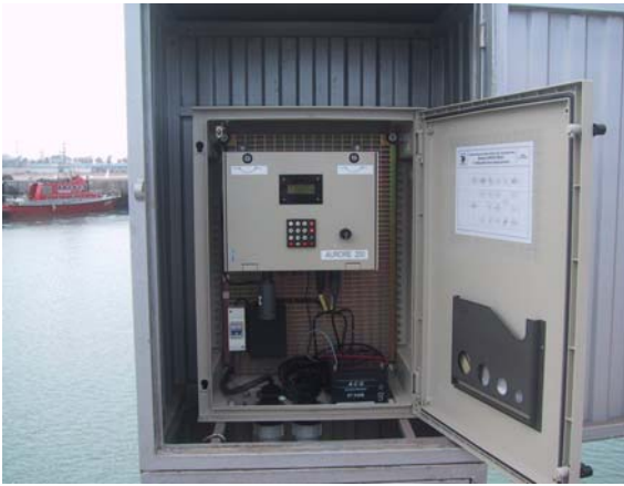
Figure 20, Mohammedia DPDPM Warsh/Martech Radar Tide Gauge. Data cartridge is the grey cylinder at the base of the Aurore 200 data logger.
