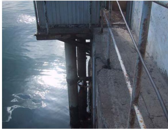
Figure 13, Old Port TG and rusting stilling wells
