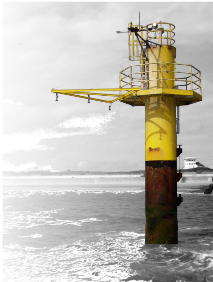
Figure 1: Radar-Array at the tide Gauge Borkum-Südstrand (S.Rüten, BfG)
