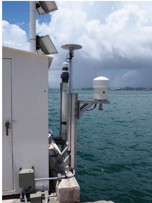
NOAA NWLON Station in San Juan, Puerto Rico showing GNSS antenna, microwave and acoustic water level sensors
