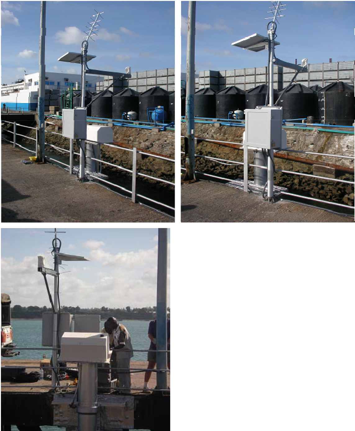
Fig 2: Photo of upgraded Mombasa tide gauge station
