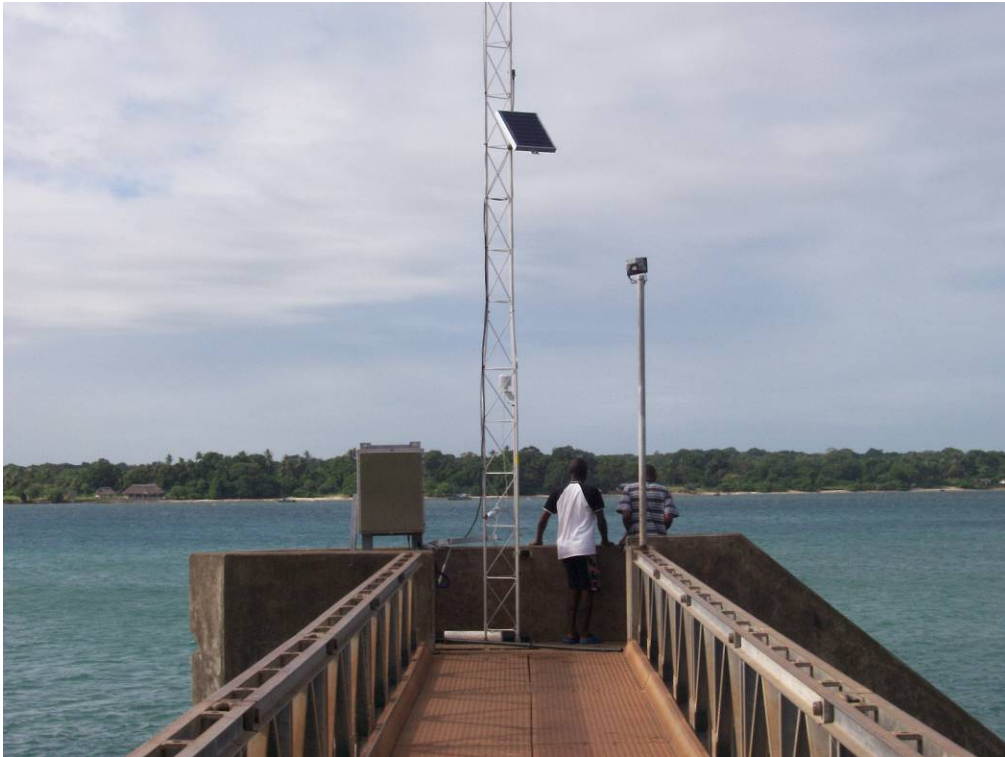
Fig5a: Wasini Island Tidal and Automatic Weather Station installed at the Old Navy Jetty
