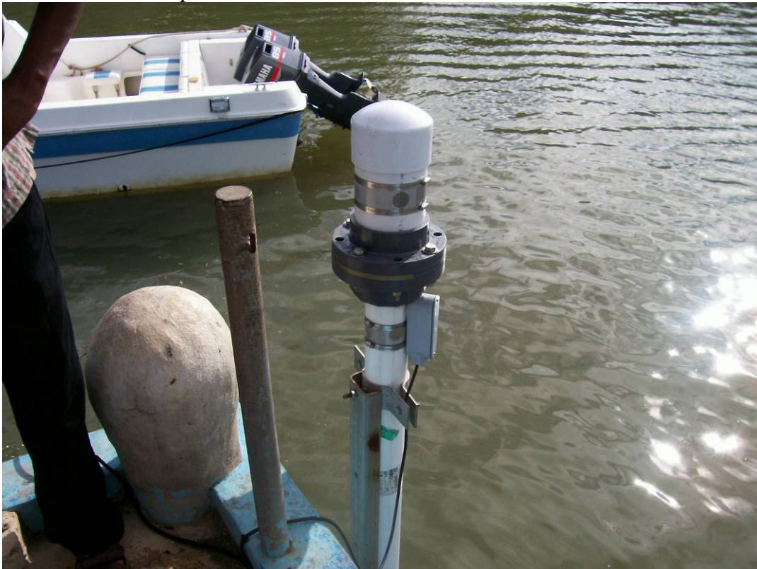
Fig 6b: Stilling Well of tide gauge at New Fisheries Jetty in Lamu Island.
