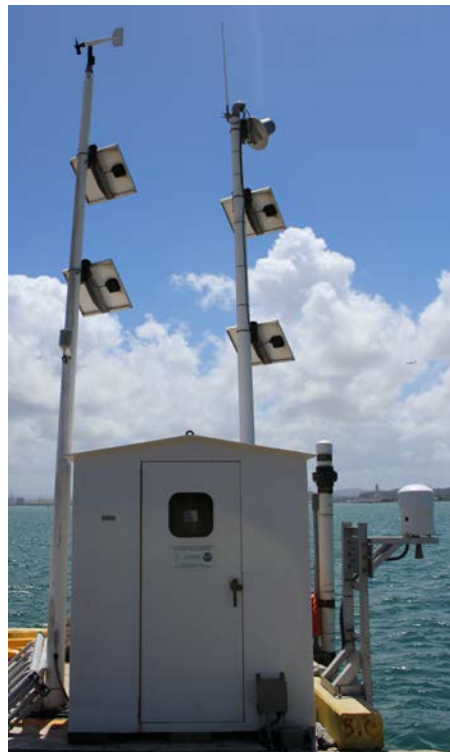
NOAA NWLON Station in San Juan, Puerto Rico with both acoustic (in back) and microwave sensors installed
