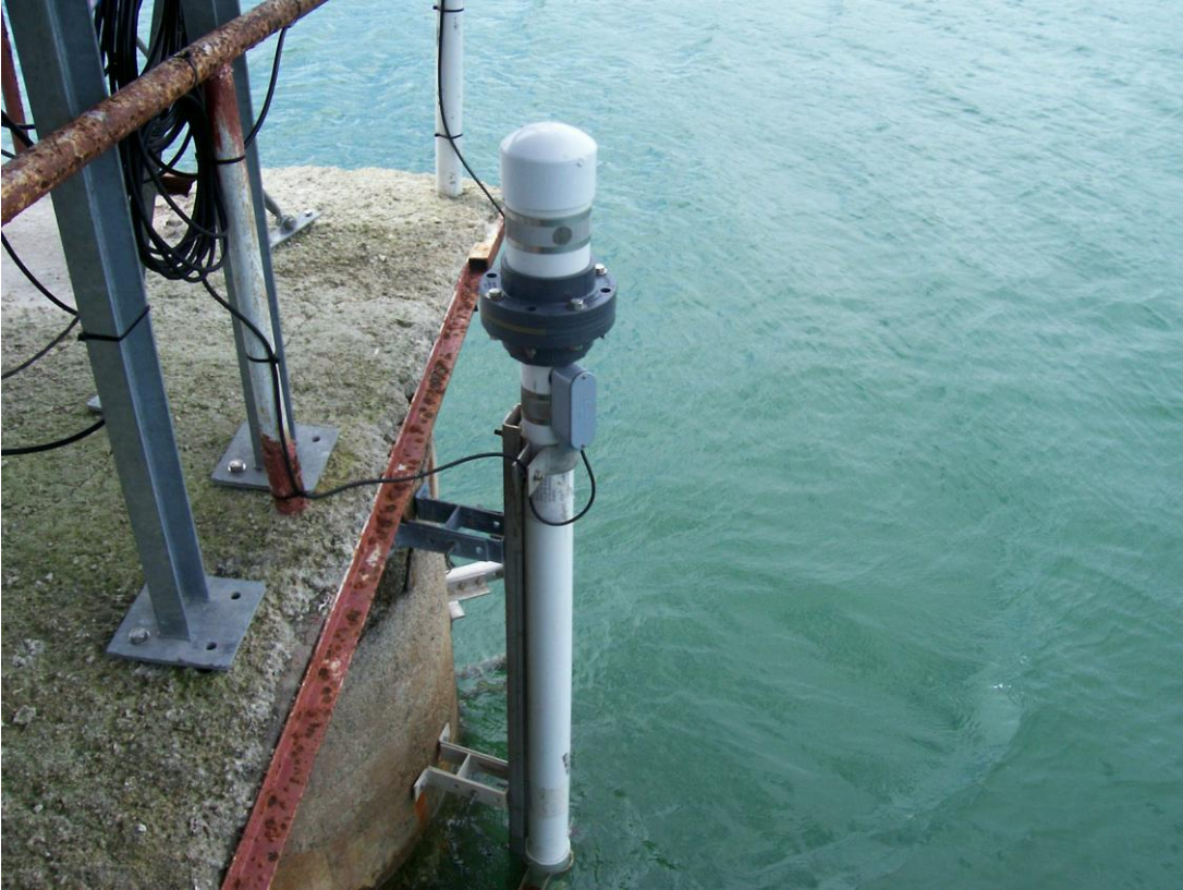
Fig 4a: Stilling well of the tide gauge at the Old Jetty of Kilifi Mnarani club.
