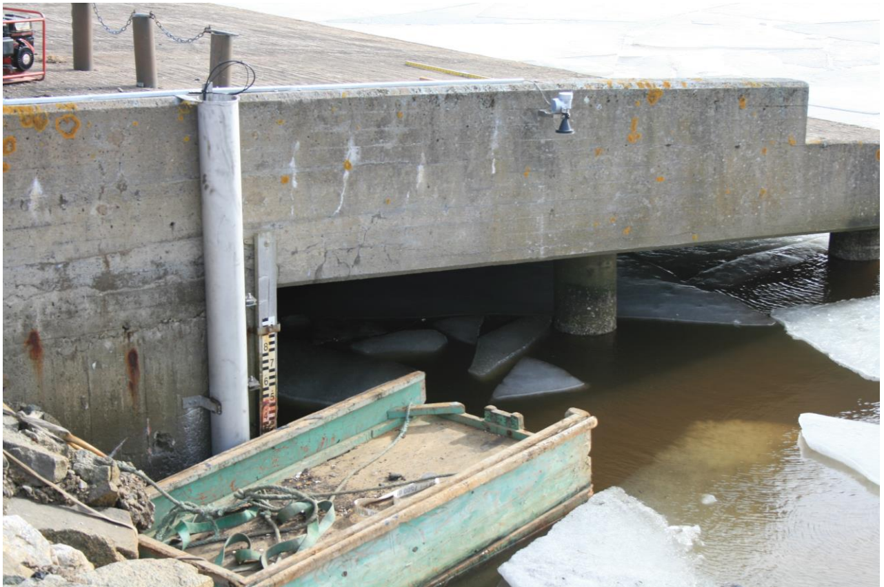
Figure 10. A mobile sea level station, which consists of a bubble-sensor (to the left) and radar sensor (to the right). During periods with ice conditions, the data from the radar sensor are neglected.
